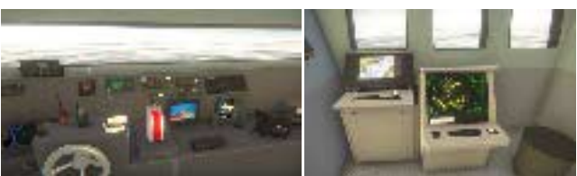
Shipboard electric equipment
